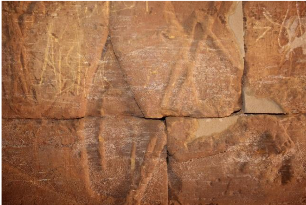
Wet Sandstone Blocks and Presence of Salt in Beg. N. 12.
